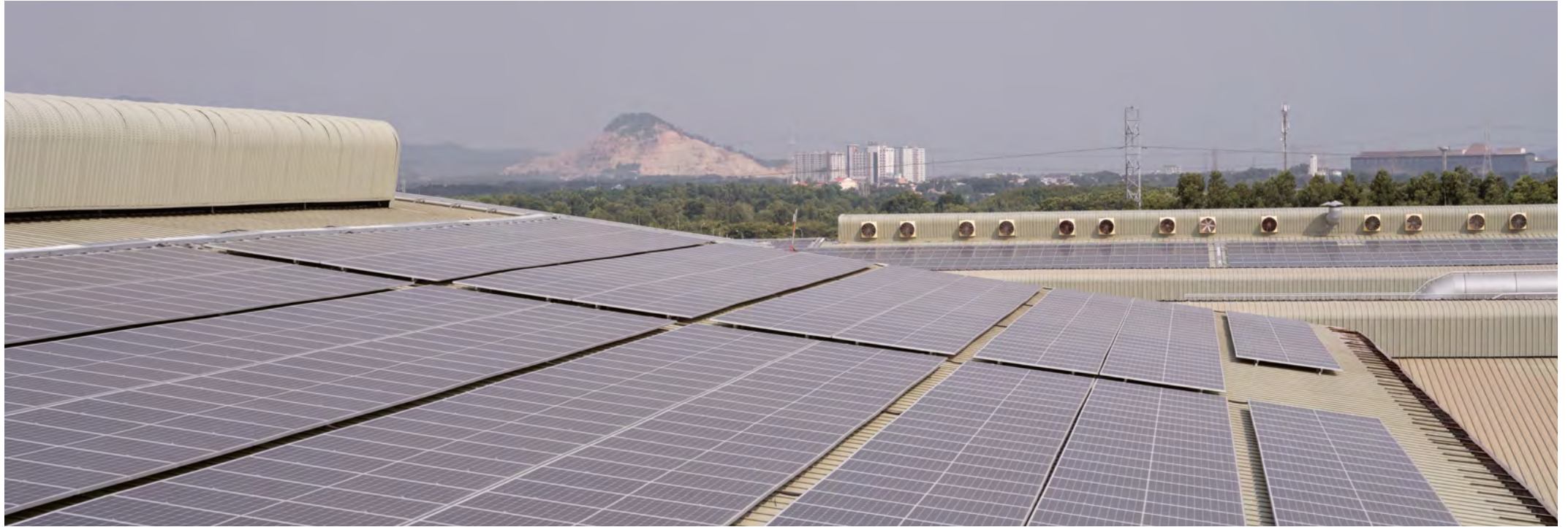
Solar panels on Eclat facility, Vietnam
