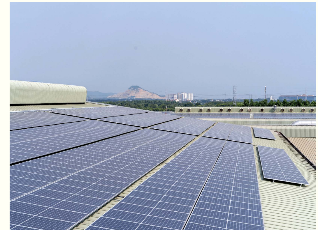
Solar panels on a supplier facility, Vietnam.
